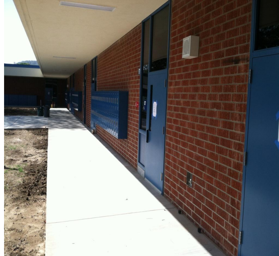
Modernized Building Exterior New Lockers, ADA Compliant Flatwork, Stucco, Paint, New Doors & Hardware
